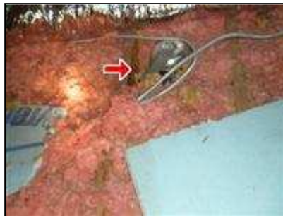
9.0 Picture 4 Insulation Voids
