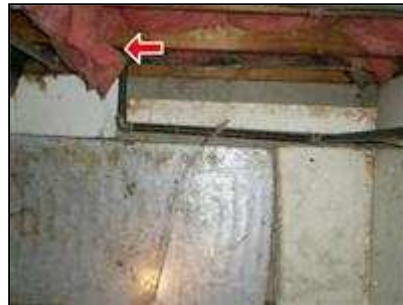
9.4 Picture 2 Loose Insulation
