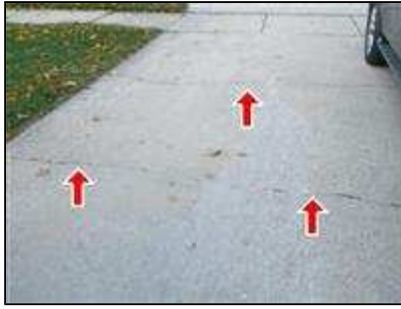
2.5 Picture 2 Cracks in Driveway
