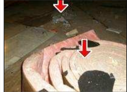
4.3 Picture 7 Insulation and Debris
