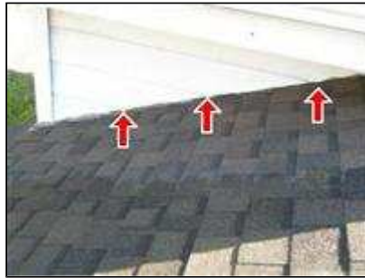
1.1 Picture 1 Sloppy Workmanship
