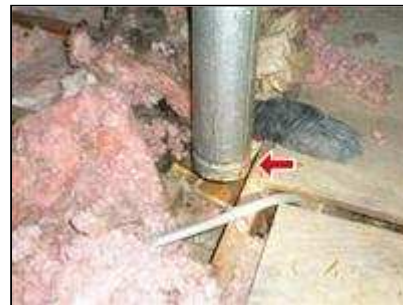
4.3 Picture 2 Abandon Flue Pipe
