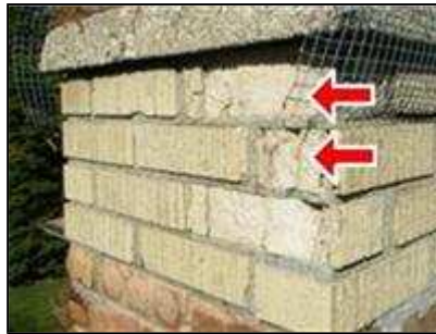
1.2 Picture 1 Spalling Briick
