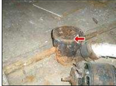
6.3 Picture 1 Open Line or Missing Vent Connection
