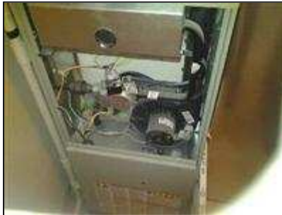
7.1 Picture 1 Dust Covered Furnace
