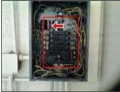
5.2 Picture 1 Federal Pacific/Stab-Loc Panel
