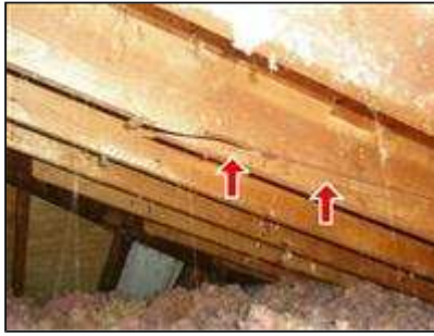
3.1 Picture 1 Cracked Rafter
