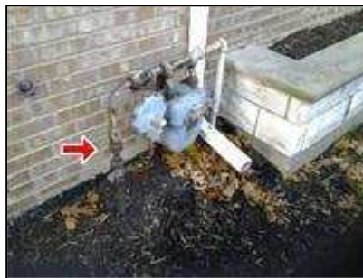
6.4 Picture 2 Main Gas Shutoff
