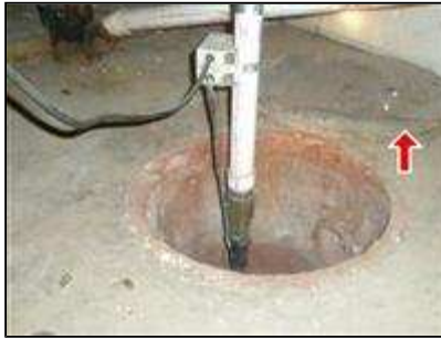
6.5 Picture 2 Cover Needs to be Installed
