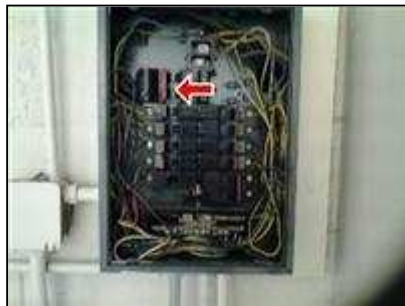
5.1 Picture 1 Main Disconnect
