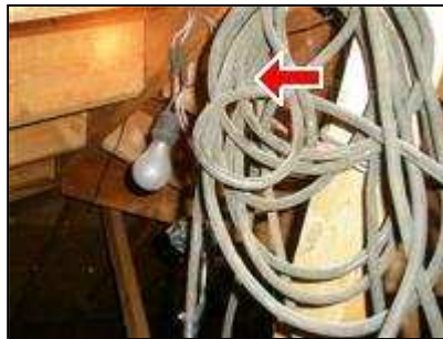
4.2 Picture 1 Unsafe Extension Cord
