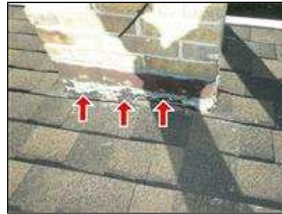
1.1 Picture 2 Sloppy Workmanship
