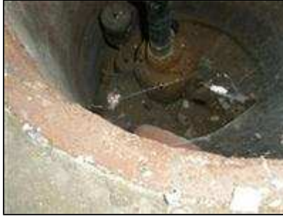
6.5 Picture 1 Dry Sump Pump
