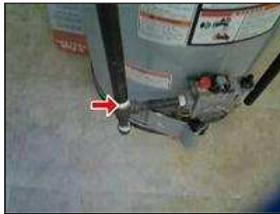
6.4 Picture 1 Gas Leak on Water Heater Connection
