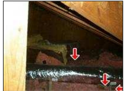
9.0 Picture 3 Insulation Voids
