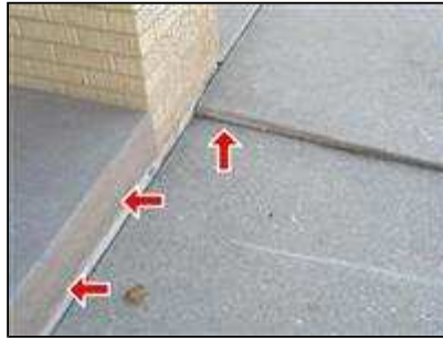
2.4 Picture 3 Step Height and Trip Hazard
