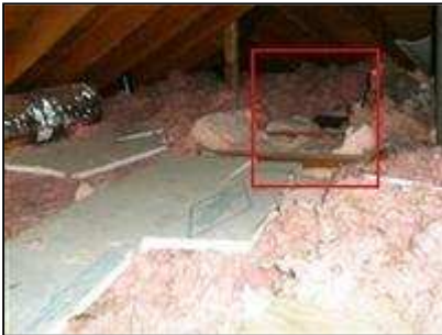
9.0 Picture 1 Insulation Voids
