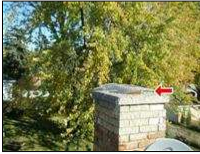
1.2 Picture 2 Screen on Chimney Flue
