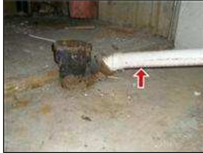
6.3 Picture 2 Drain Line from Kitchen Sink
