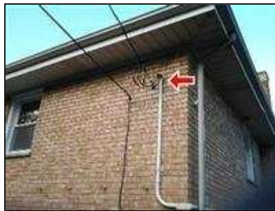
5.0 Picture 1 Service Entrance Wires
