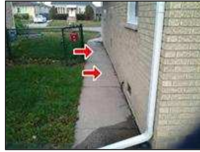
2.4 Picture 2 Settled Sidewalk
