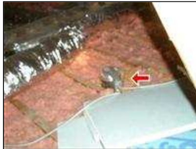
9.0 Picture 2 Insulation Voids
