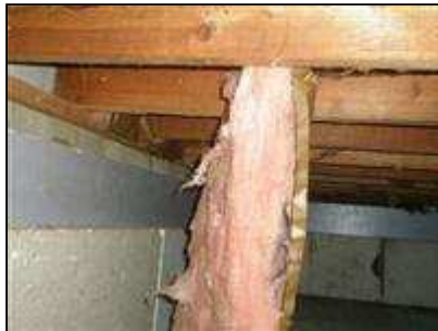
9.4 Picture 1 Falling Insulation
